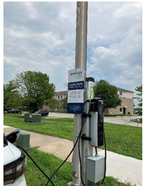
Figure 17. EV charger installation at 9701 N. Shannon Ave, Kansas City, MO 64513
